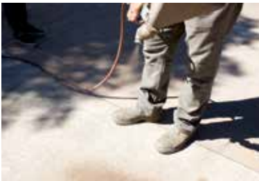
The Stylepave Overlay is spray applied by hand with a compressed air controlled hopper gun.
